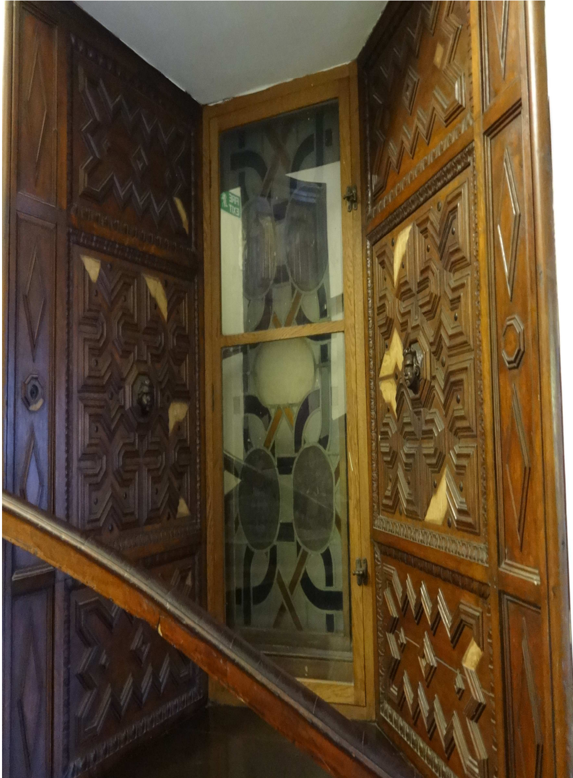
The first window on the right of the staircase was damaged during alterations The centre missing panel had The head of JOHN the BAPTIST On a Plate
